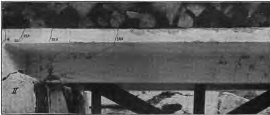
FIG. 187.—Beam II, Cracks and Rupture in the vicinity of the intermediate support.
