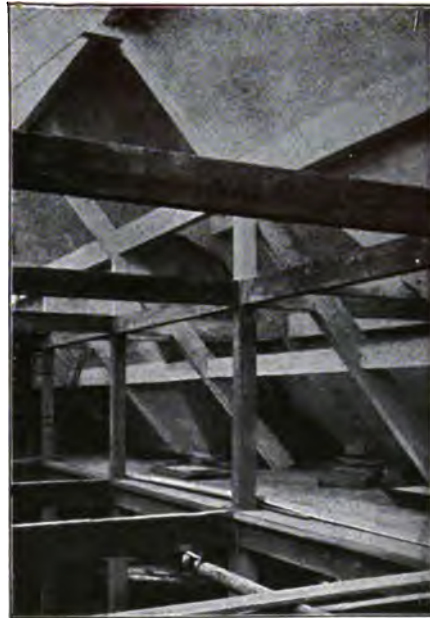
FIG. 232.—Reinforced concrete roof supports in the building of the “Münchenen Neuesten Nachrichten.”
