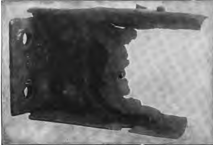
FIG. 283.—Rusting of a main girder by locomotive gases.
