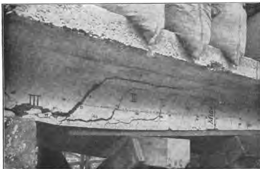
FIG. 120.—Failure cracks in the vicinity of the points of support of a T-beam reinforced with straight Thatcher bars.
