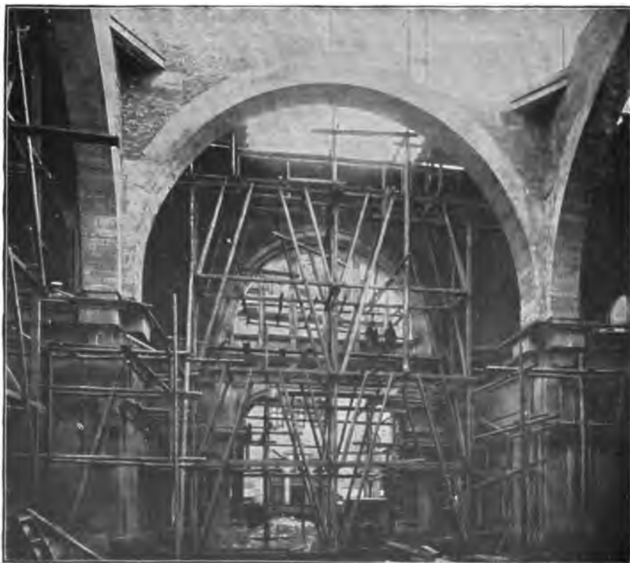
FIG. 249—Reinforced concrete semi-circular arches in the cupola of the new station in Nürnberg.
