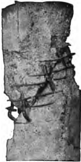
FIG. 72.—Failure from shear. (Spiral broken.)
