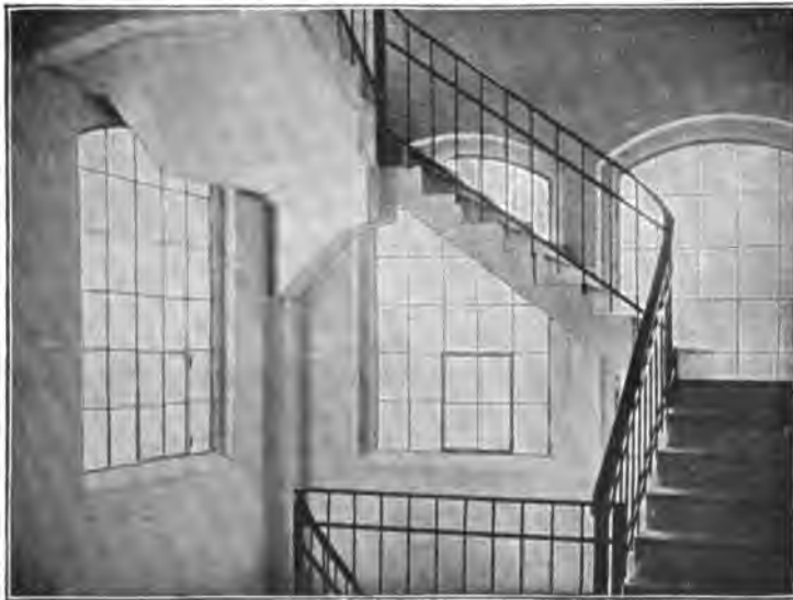
FIG 243 —Reinforced concrete stairs in the storehouse of the National Railway, Elberfeld in Opladen.
