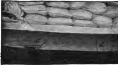
FIG. 170.—Bursting effect of loose diagonal stirrups.
