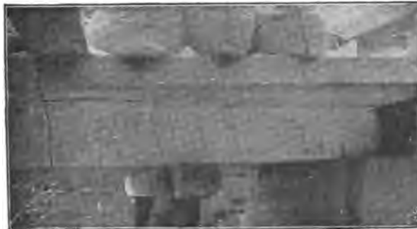
FIG. 135.—Beam I, cracks in the end supplied with stirrups, at the breaking load.
