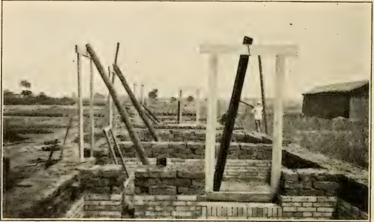
FIG. 75. - Foundation of dwelling, consisting of hard-burnt brick; balance of wall to be sun-dried earth brick, seen in Fig. 74.
